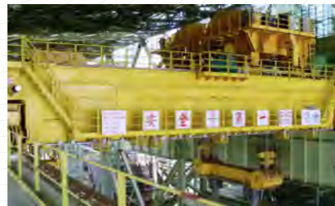
360t铸造起重机 360t ladle crane
