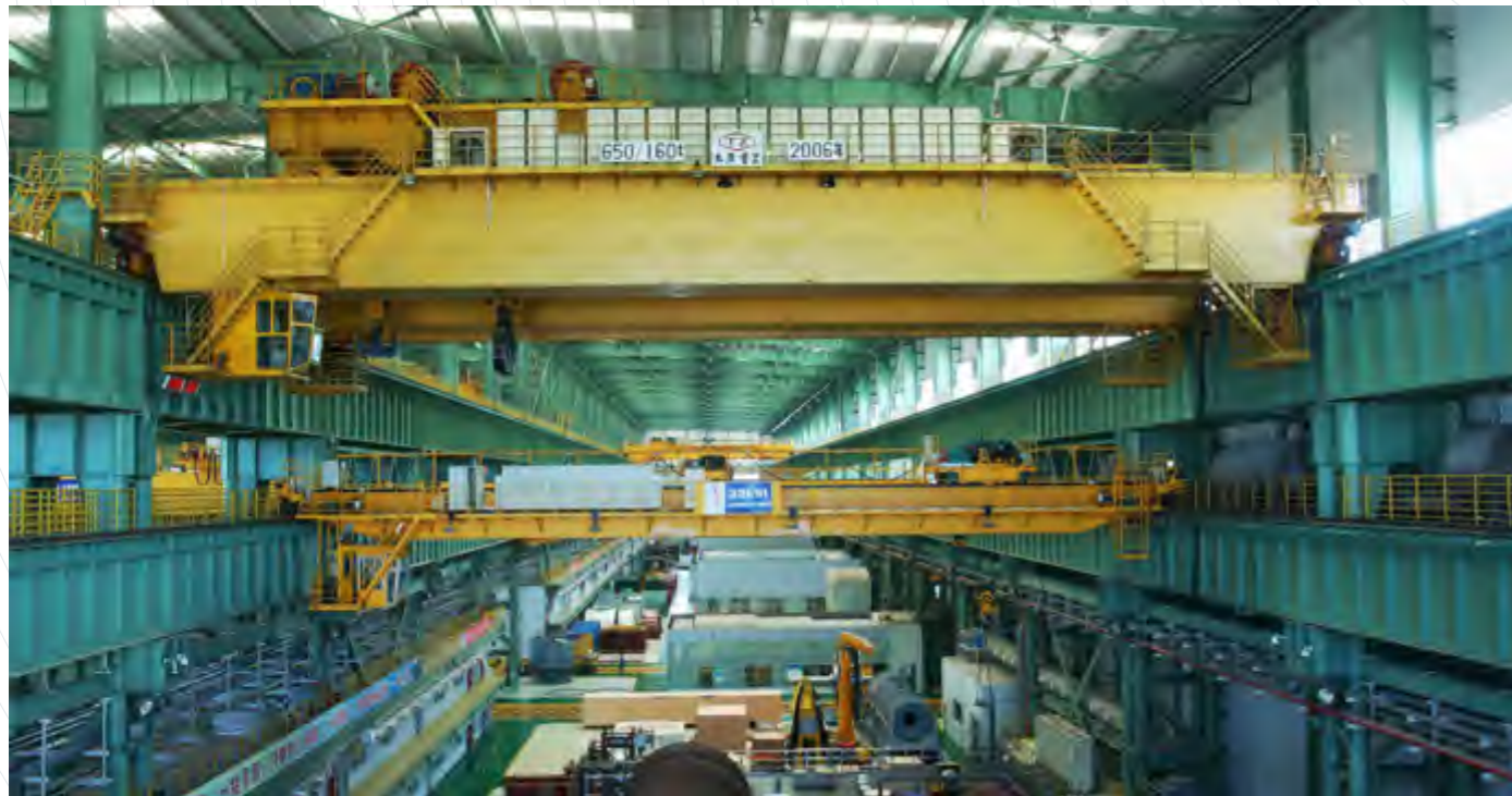
650t/160t 桥式起重机 650t/160t Bridge Crane
