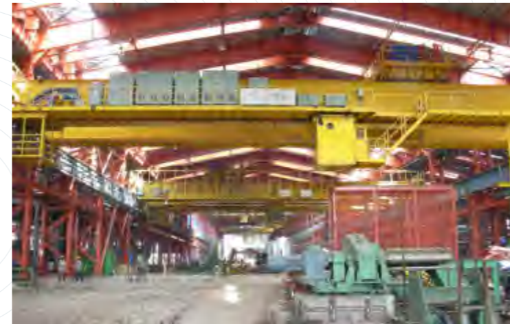
75t 桥式起重机 75t Bridge Crane
