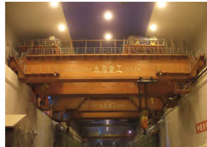
500+500t 桥式起重机 500+500t Bridge Crane
